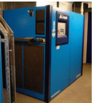
Above and top right: Rohde & Schwarz's switch to a DH oil-free compressor quickly paid for itself
